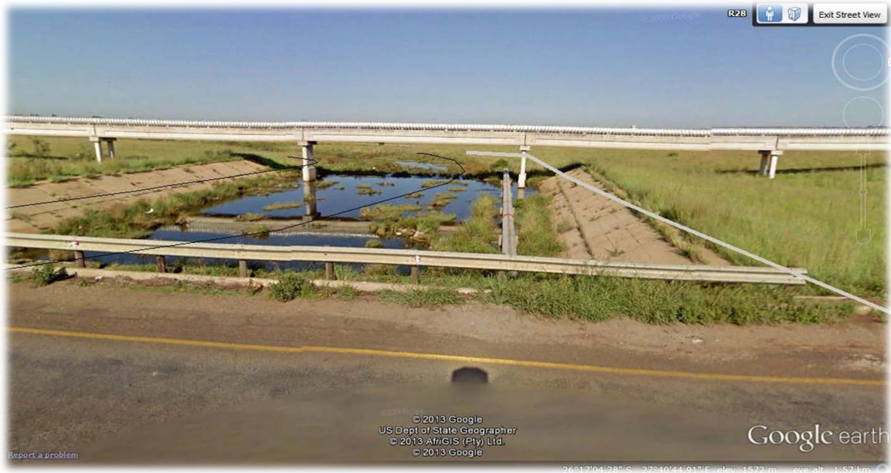
Photo E2.8: The start of the +/- 30 km 1 metre diameter pipeline that conveys water from Donaldson Dam over the dewatered dolomite compartments to prevent filling of compartments and flooding of mines.
