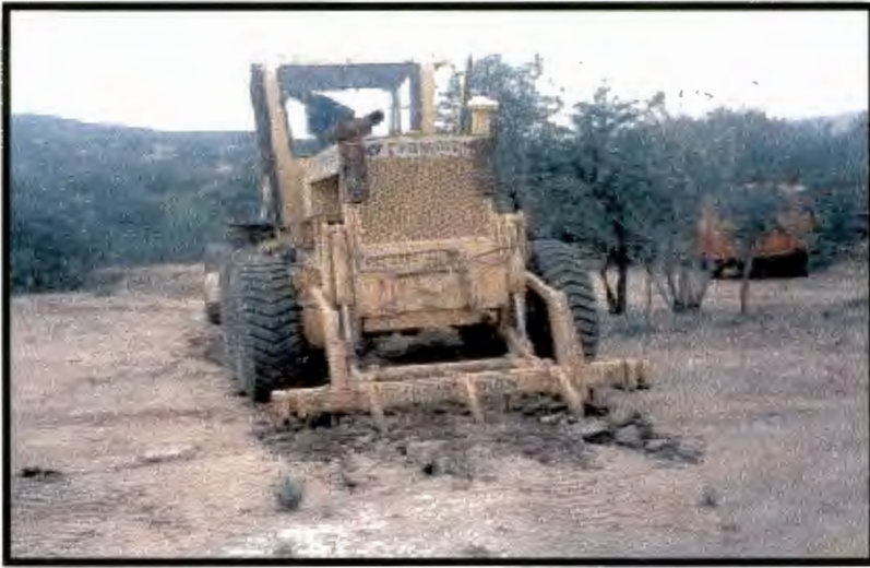
Figure 3.3. A grader with a ripper attached was used to rip the soil at a depth of 15cm to 20cm along the contours.
