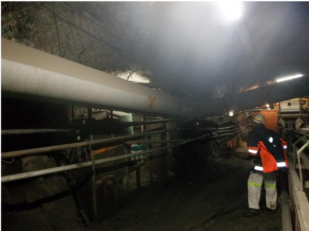
Figure 22: Main line 90° bends over conveyor
