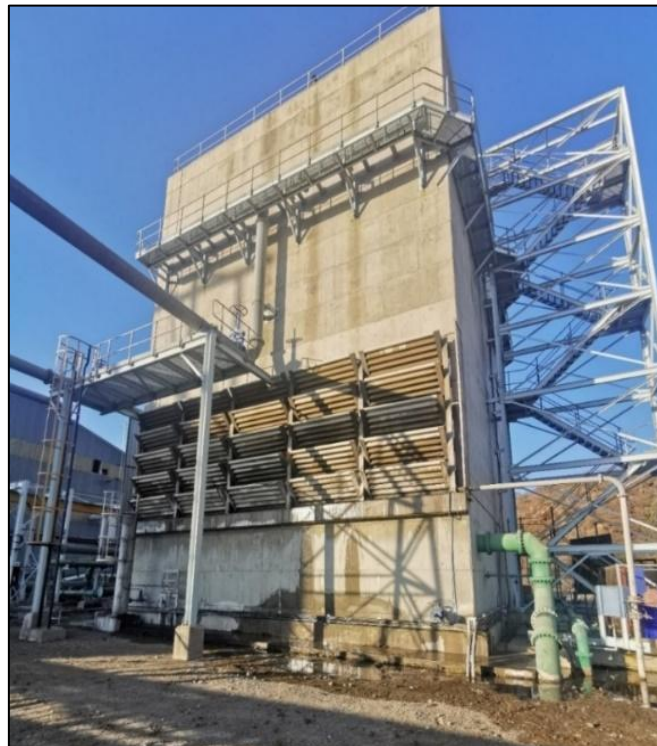
Figure 9: Surface cooling tower [Taken by author]
