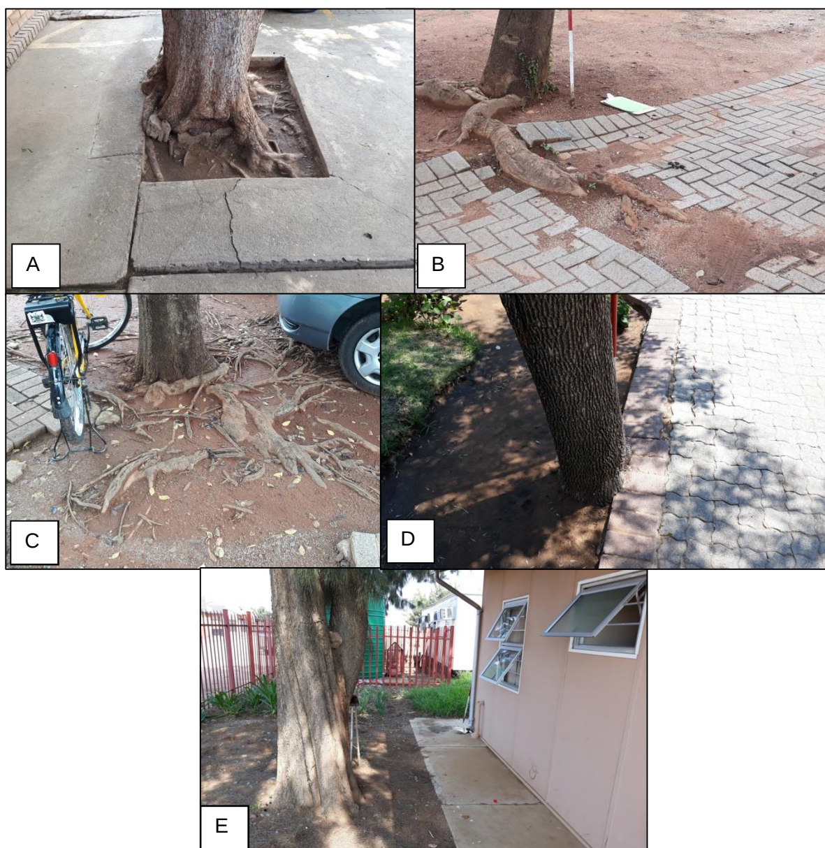
Figure 3-27: A. A Fraxinus velutina that was causing root damage to the paving at the Boiki Tlhapi clinic. B. A Brachychiton populneus that had lifted paving stones with its roots at the Jouberton clinic. C. A Celtis sinensis that had lifted paving stones with its roots at the Jouberton clinic. D. A Fraxinus velutina that could lift paving in the future at the Leeudoringstad clinic. E. A Casuarina cunninghamiana that could potentially be causing or cause damage at the Empilisweni clinic.
