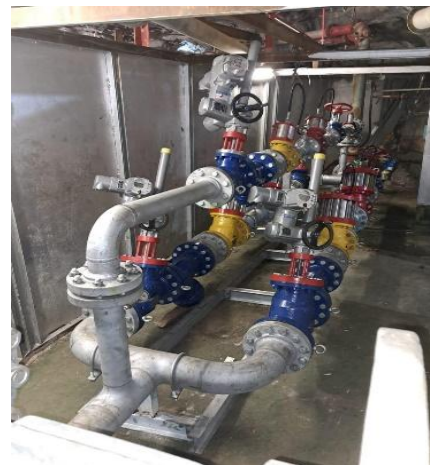
Figure 3-38: Newly installed 200 NB ratio valve station 18
