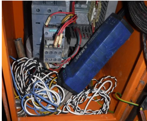
Figure 3-11: Portable power logger
