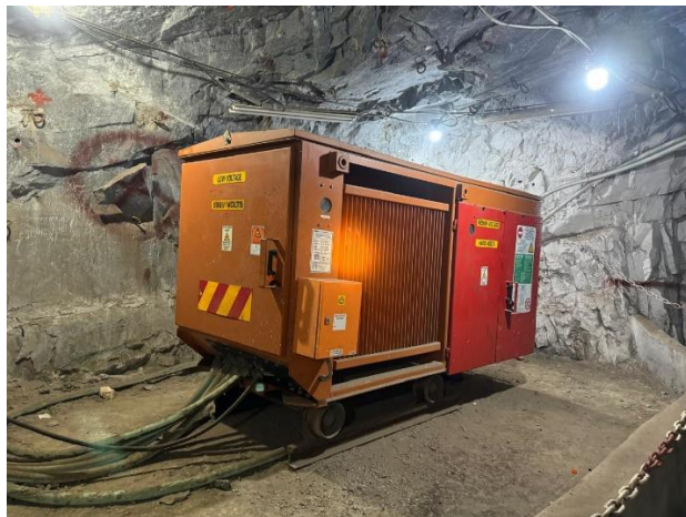
Figure 3-37: Newly installed 630 kVA mini-substation 17
