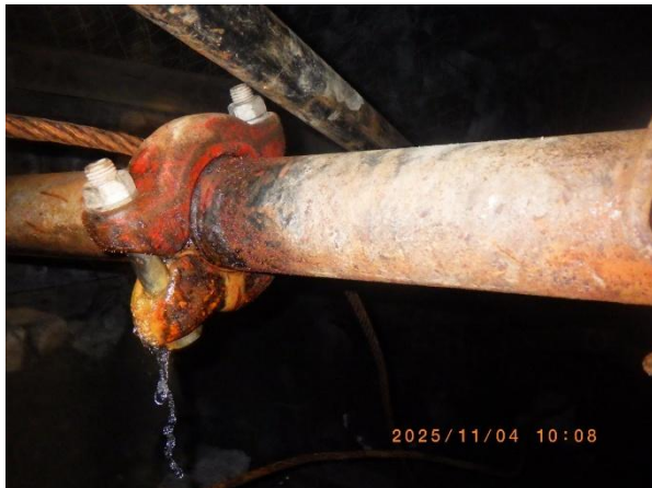
Figure 3-71: Hydropower high-pressure pipe connection leak 31
