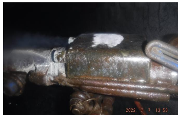
Figure 3-46: Frost formation near the outlet port 25
