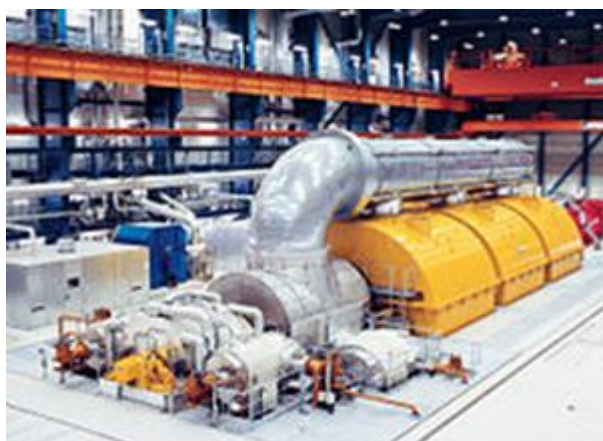
Figure 1: A power plant turbo generator cooled with hydrogen [2].
