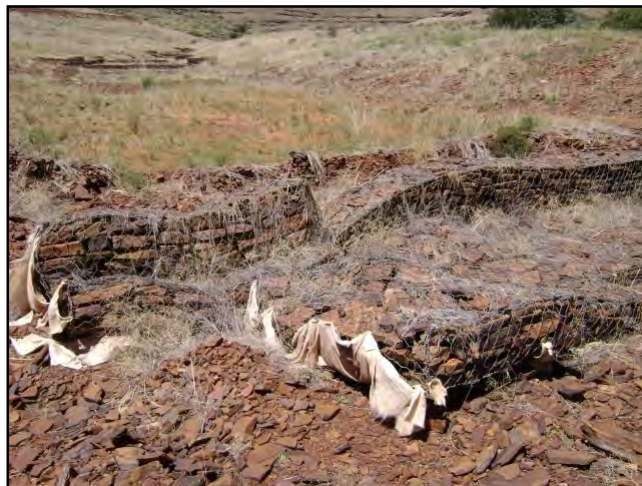
Figure 3-15: Damaged retaining weir 2 in the Northern Cape Province, where the gabion structure was damaged by floods.
