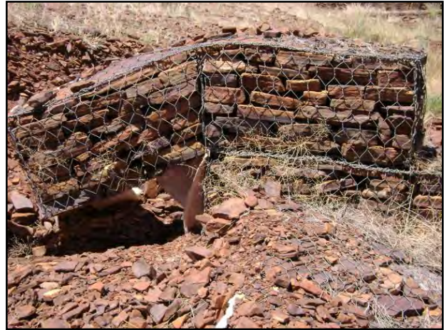
Figure 3-14: Damaged retaining weir 1 in the Northern Cape Province at the Kuruman-East asbestos mine.
