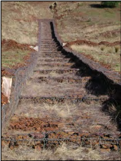
Figure 3-13: Damaged waterway in the Northern Cape Province
