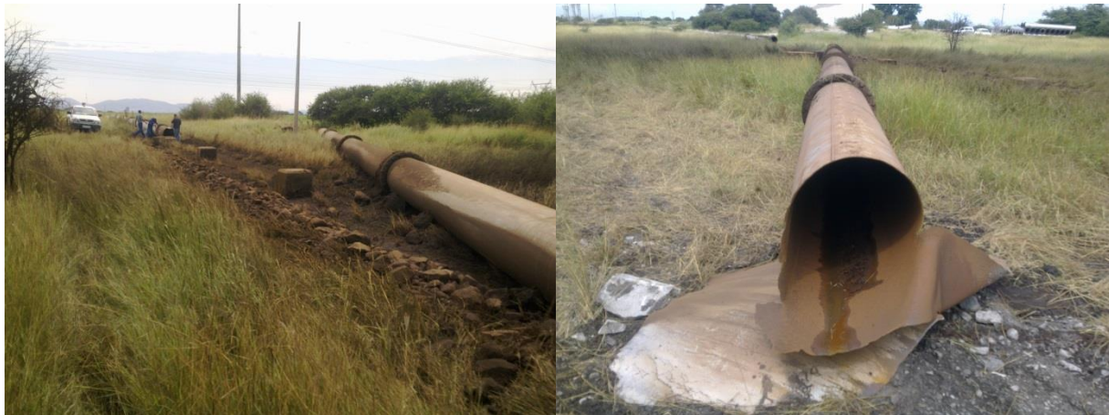
Figure 11: Photos of a burst compressed air pipeline at a platinum mine
