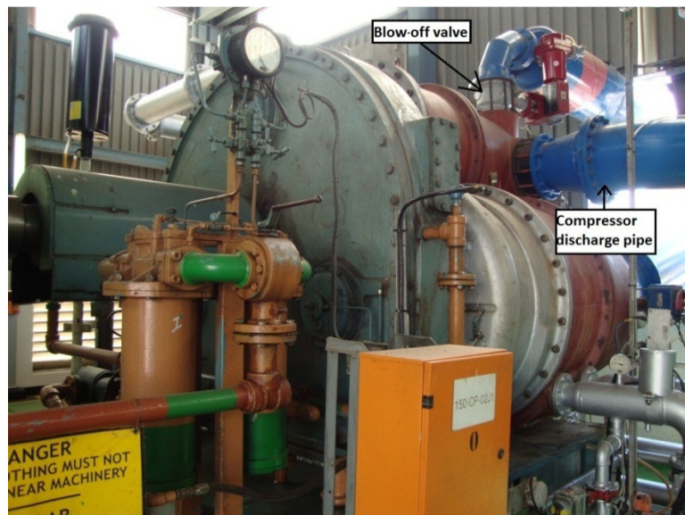
Figure 13 – Photo showing a blow-off valve on a centrifugal compressor 13
