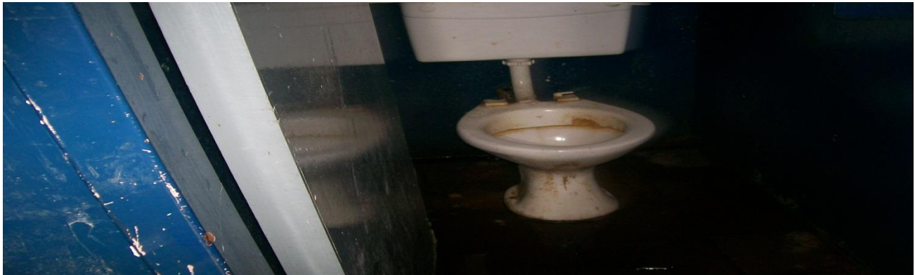
Figure 4.2: Unclean toilet in school C
