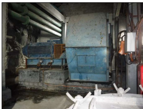
Figure 3-25: Condenser pond 5 booster fan
