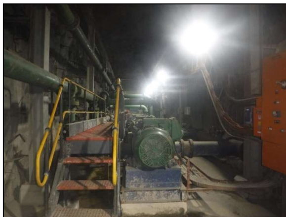
Figure 3-24: Condenser pond 5 pumping station
