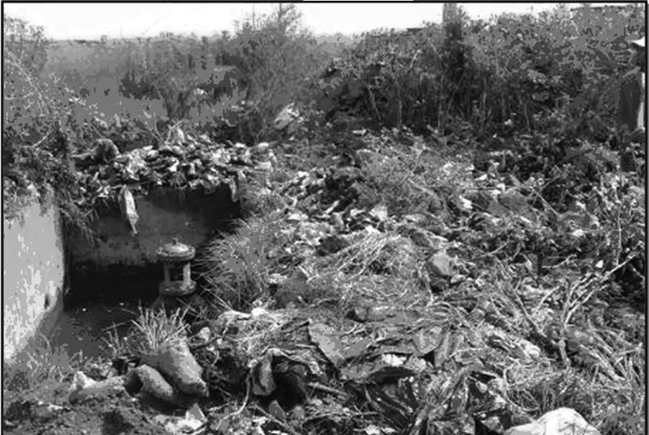
Figure 6: Identification of missing valve and chamber after cleaning
