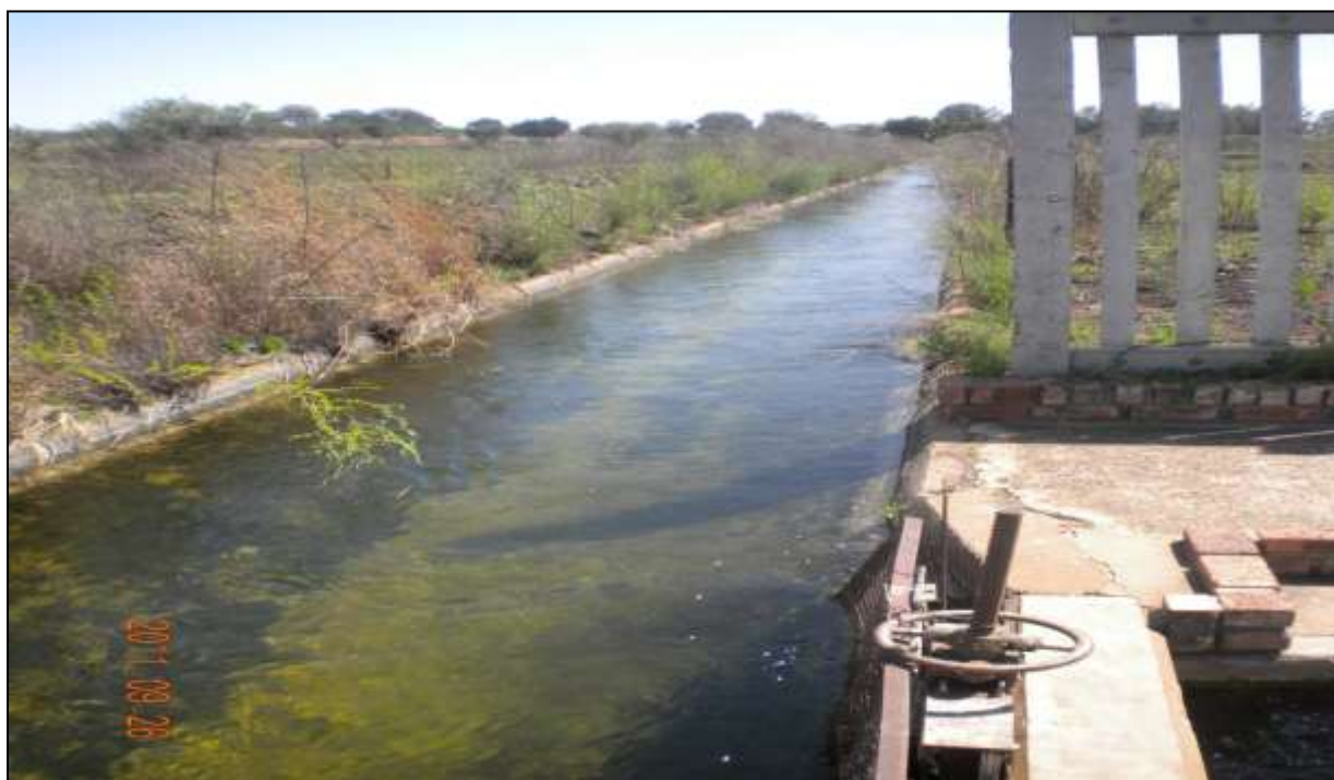
Photo 8: Open-on-top cement canals transporting water destined for consumption by Ventersdorp residents
