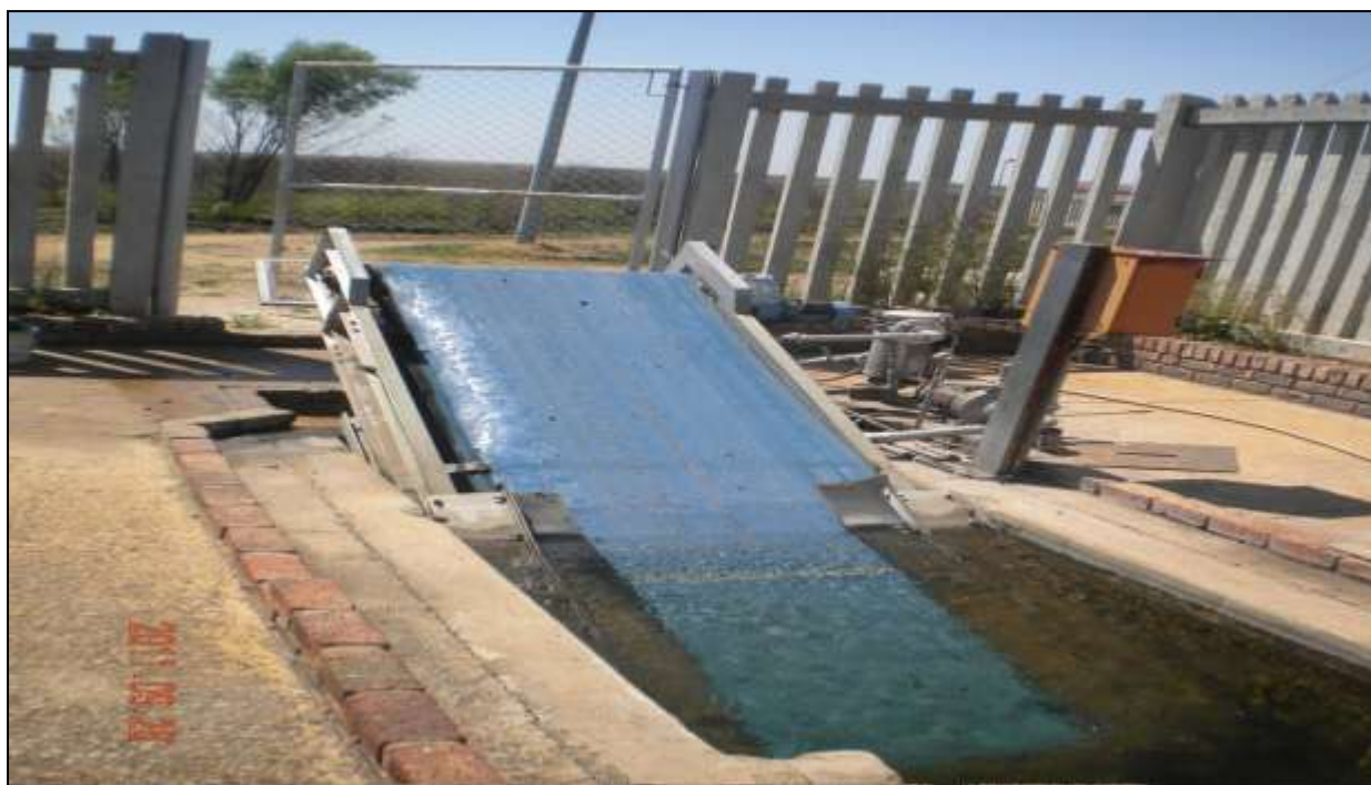
Photo 7: Water purification works at Ventersdorp Local Municipality
