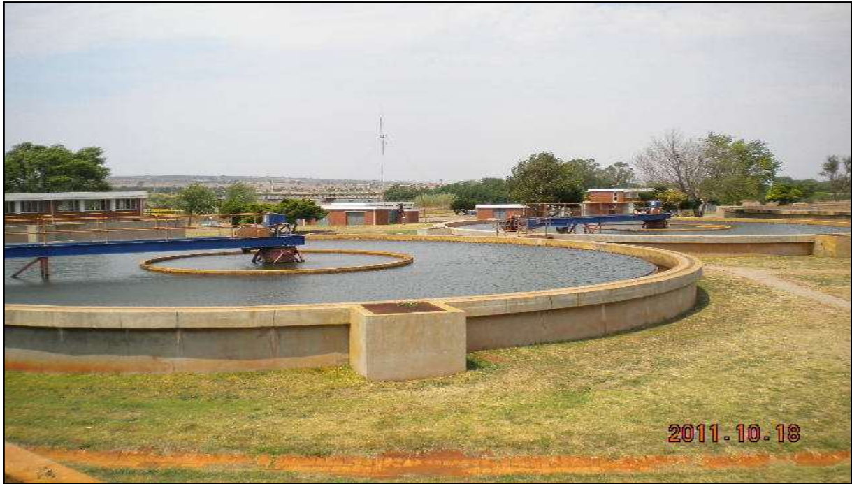
Photo 4: Water treatment works of Tlokwe City Council
