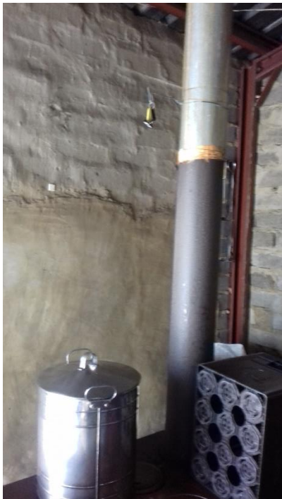
Non insulated inside
