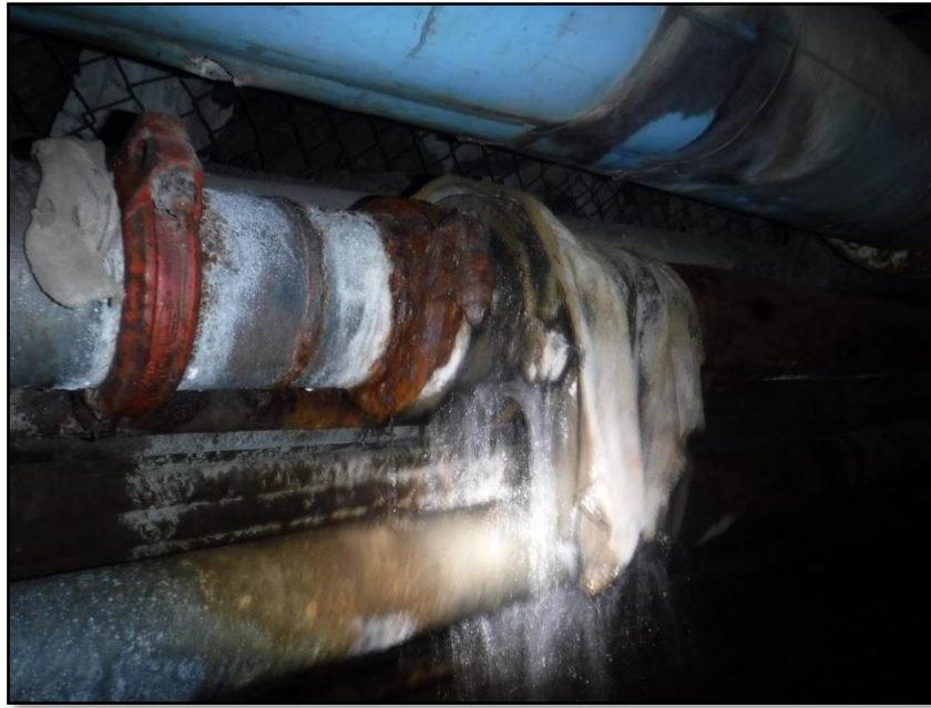
Figure 13: Failing RAW pipeline 6
