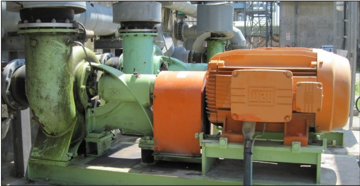
Figure 28: Typical centrifugal water pump and electric motor configuration.
