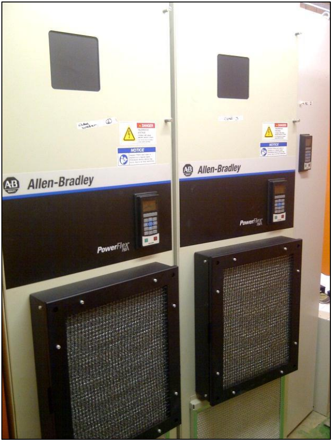
Figure 80: VSD installed on the evaporator pumps.
