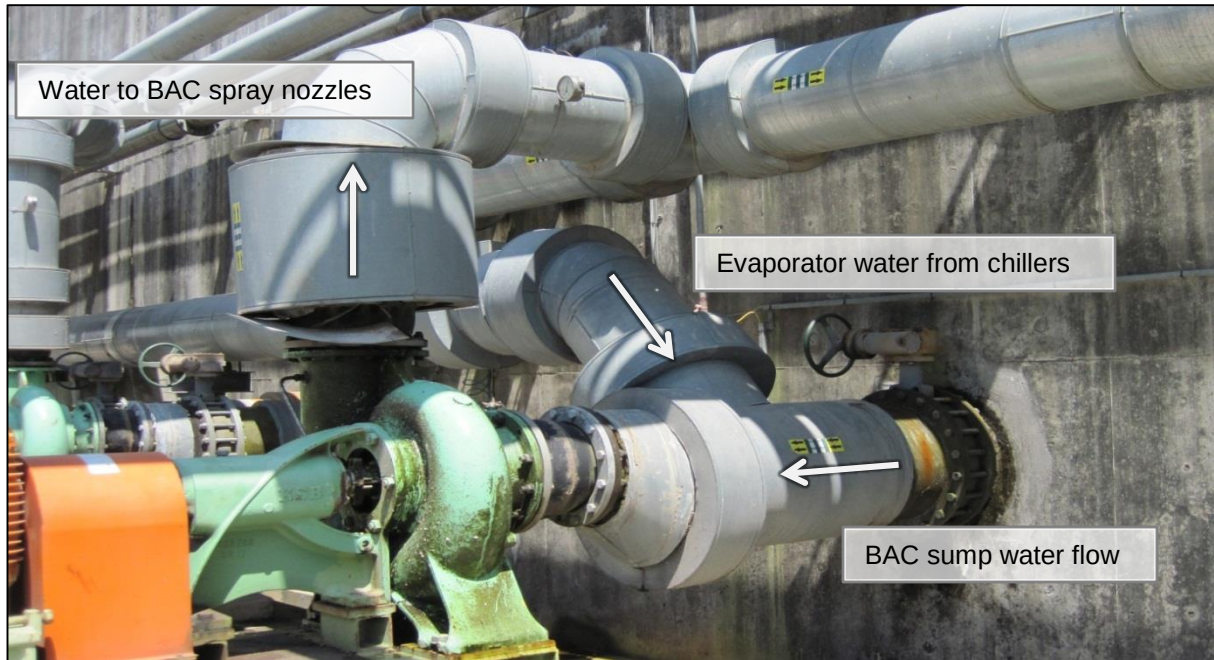
Figure 44: Mine A BAC first stage spray pump water supply and delivery network.
