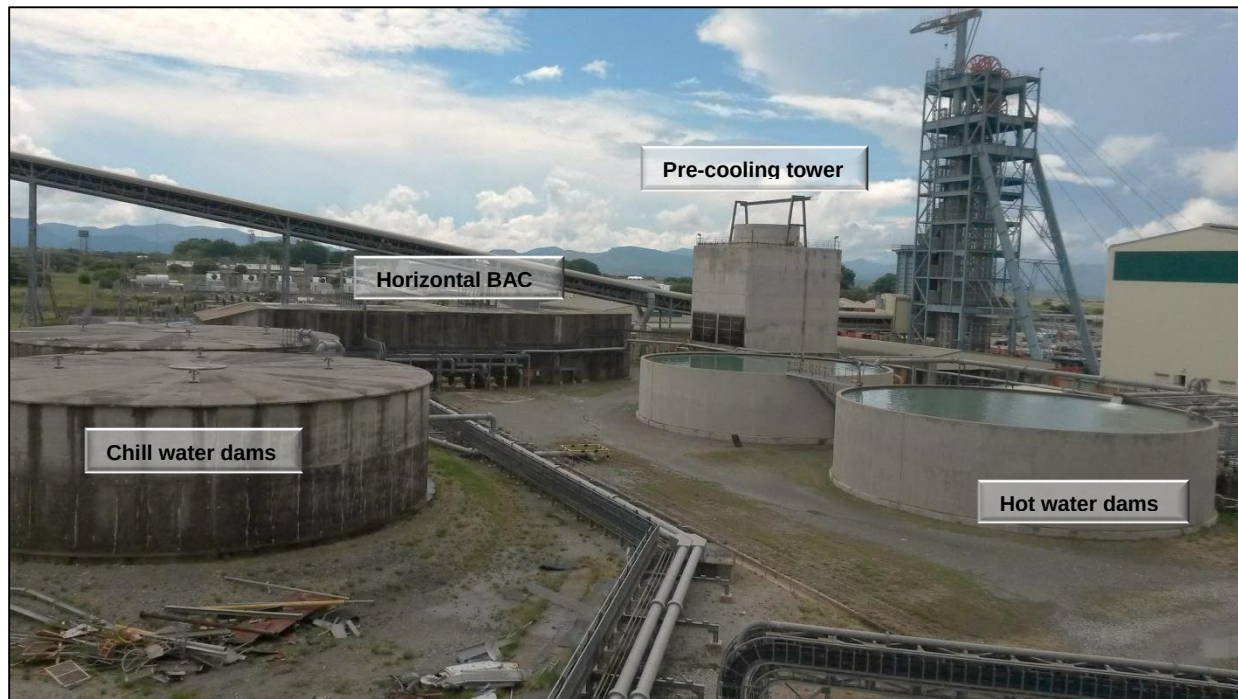
Figure 27: Surface chilled and hot water storage dams installed on a platinum mine near Thabazimbi.
