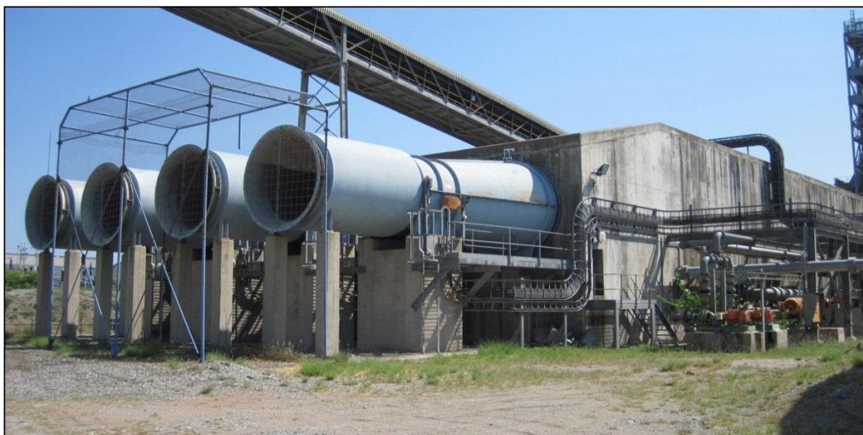
Figure 20: A multi-stage horizontal BAC used on a platinum mine near Thabazimbi.
