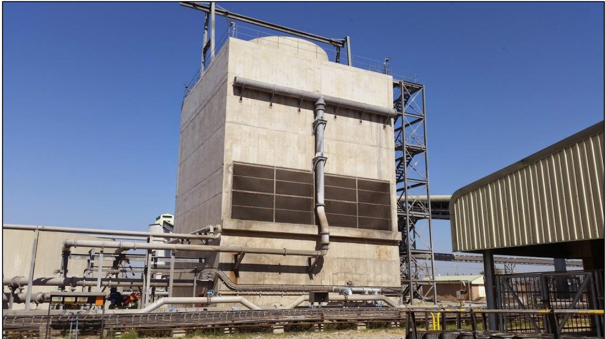
Figure 14: Mine pre-cooling tower used to pre-cool hot water from underground.
