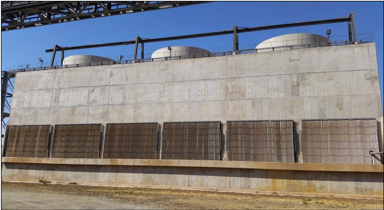
Figure 16: Mine condenser cooling towers staged next to each other.
