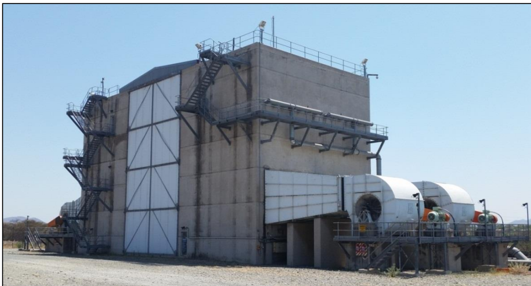
Figure 18: A multi-stage vertical BAC used on a platinum mine near Northam.
