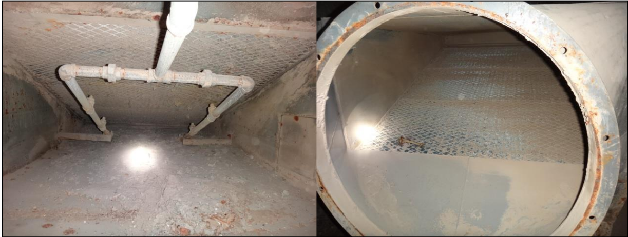
Figure 24: Secondary ventilation cooler compact heat exchanger.
