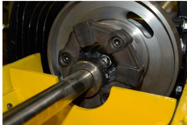
FIGURE 7.8: RADIAL CENTAFLEX COUPLING BOLTS RIPPED OUT OF HUB.
