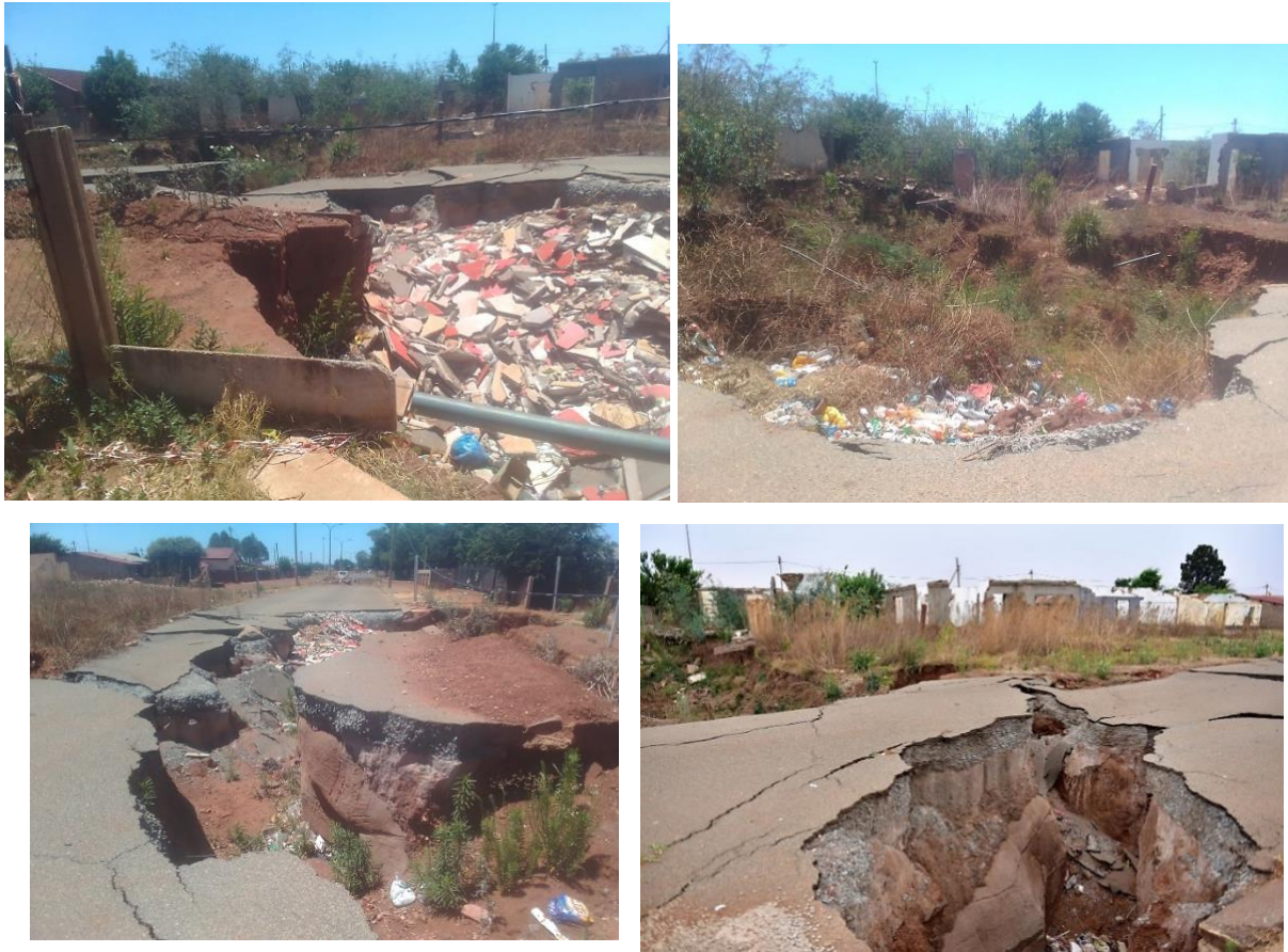
Images 5.4-5.7: Typical sinkholes in Khutsong in recent times. 117
