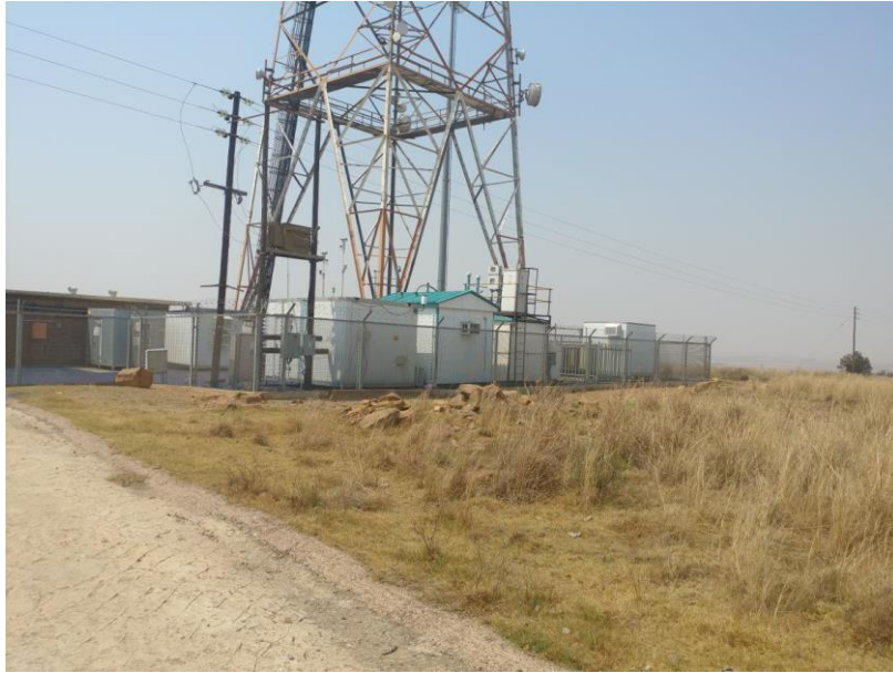
Figure 3-5: Elandsfontein air quality monitoring station.
