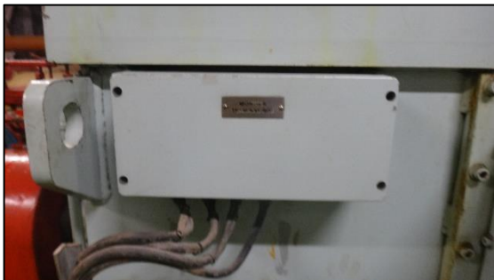
Figure 66: Motor winding temperature junction box
