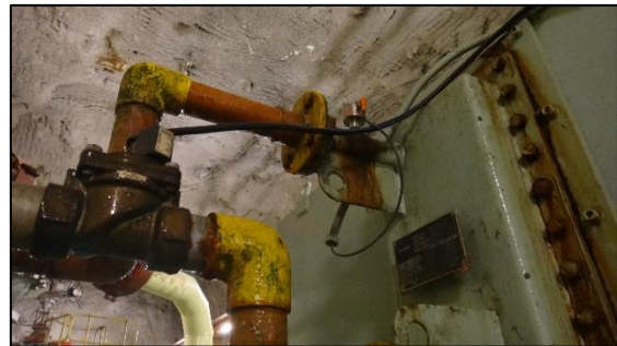
Figure 65: Motor cooling water flow switch
