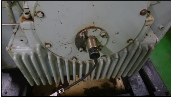
Figure 62: Motor shaft displacement switch
