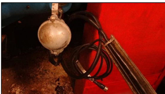
Figure 68: Pump DE bearing vibration sensor (black) and temperature sensor (grey)
