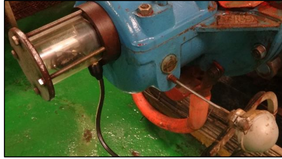
Figure 71: Pump NDE bearing temperature sensor and pump impeller displacement switch
