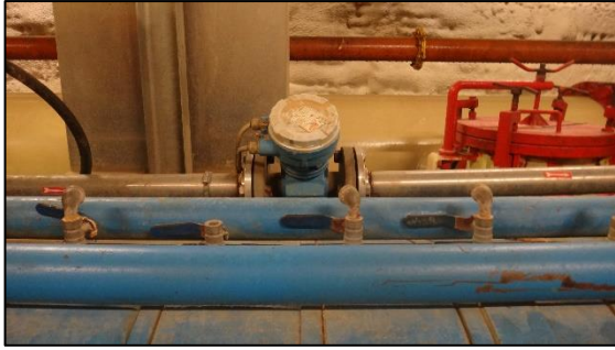
Figure 70: Pump balance disc flow sensor
