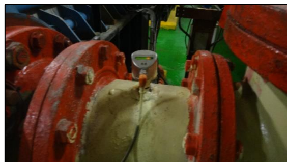
Figure 69: Pump suction flow switch
