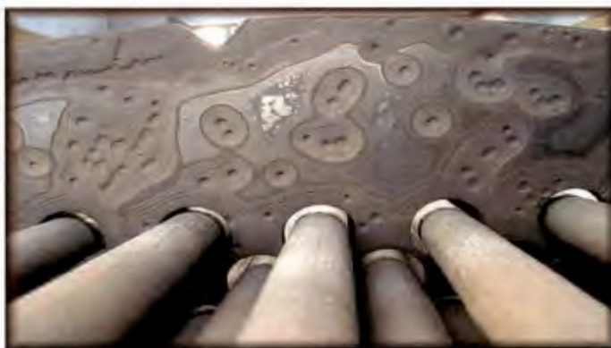
Fig. 8: Erosion corrosion of the shell side fluid in the tube and shell exchanger.
