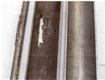
Fig. 5: Pitting on an oily water line.
