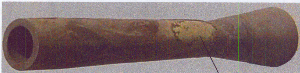
Patches of material deterioration
