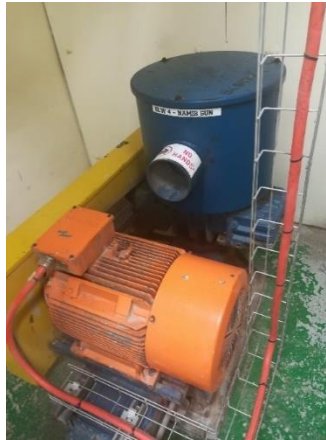
FIGURE 4 MOTOR AND BLOWER DRIVEN BY BELTS
