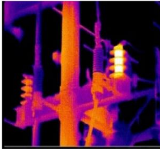
FIGURE 17 PORCELAIN INSULATION MONITORED BY INFRARED IMAGING
