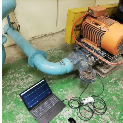
FIGURE 65 BLOWER CONDITION MONITORING WITH COMPUTER
