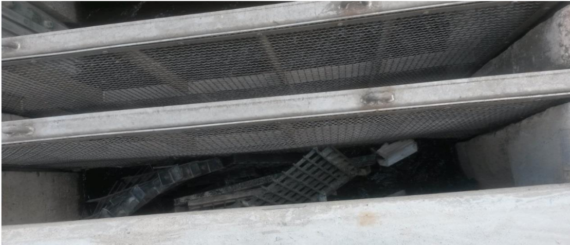
Figure 38 Blocked cooling tower screens due to broken off packing
