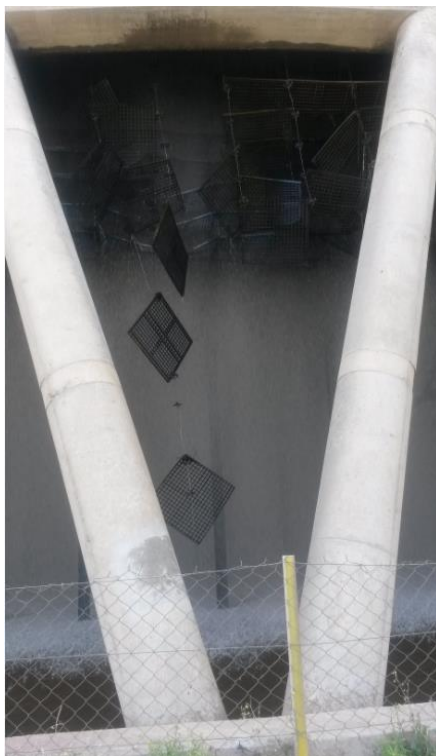
Figure 37 Broken cooling tower packing
