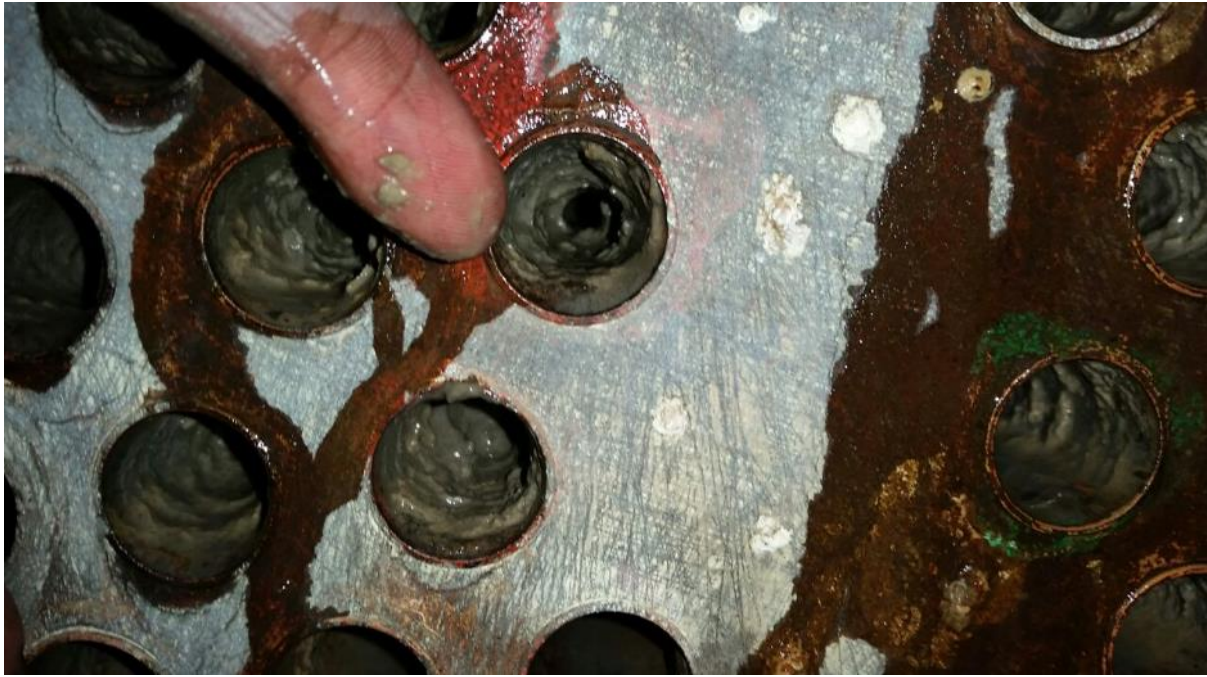
Figure 41 Image of the grey-brown sludge found inside Unit 3's condenser tubes A sample of this sludge was taken and sent for analysis.
