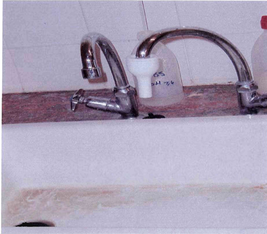
Figure A.17 Water utility supply at sink. Sink fitted in laboratory.
