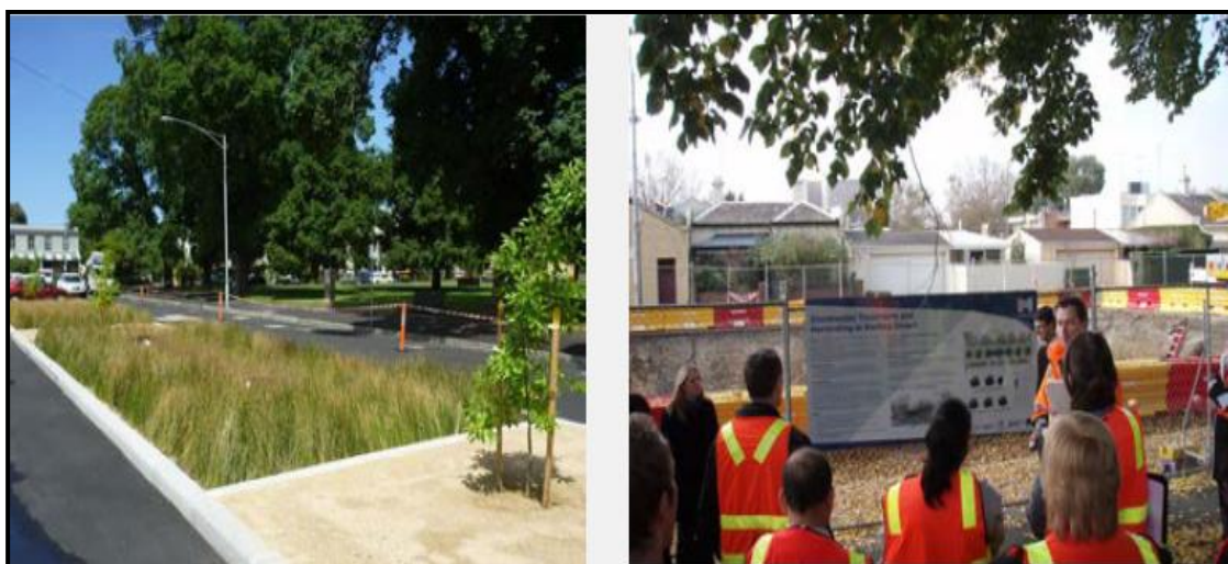
Figure 41: Biofilter median strip on Darling Street underground storage tank during construction Source: Pflidere (2012)
