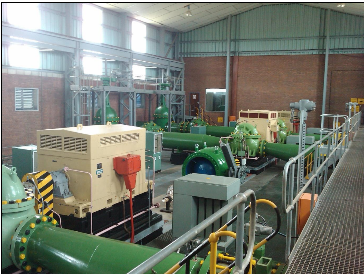
Pump-motor sets at Pump station C 9
