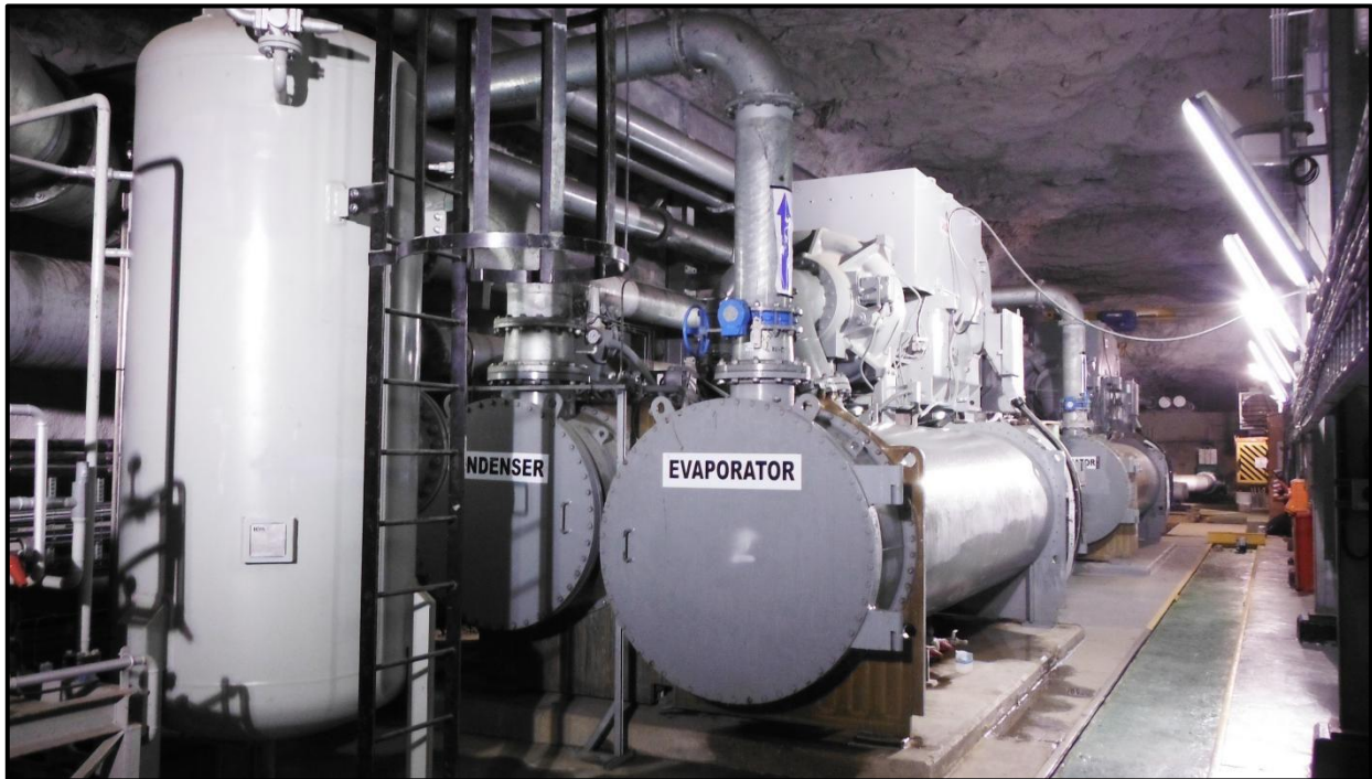
An underground refrigeration plant used to chill water 5 .
