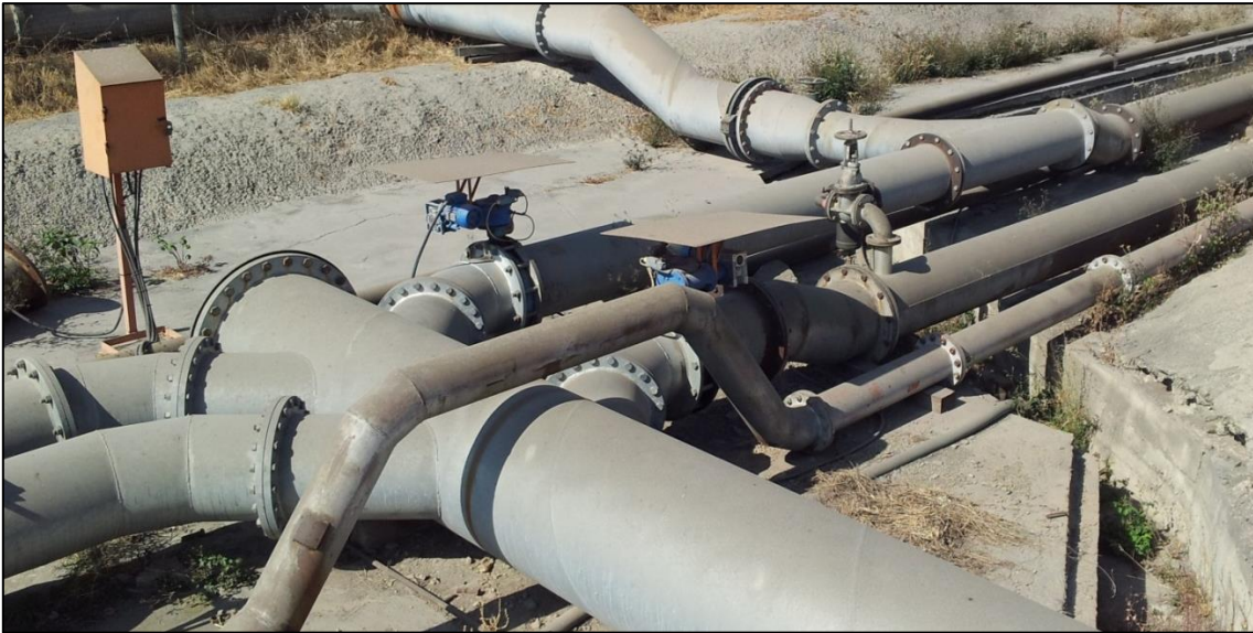
Figure 8: Compressed air network flange joints 3
