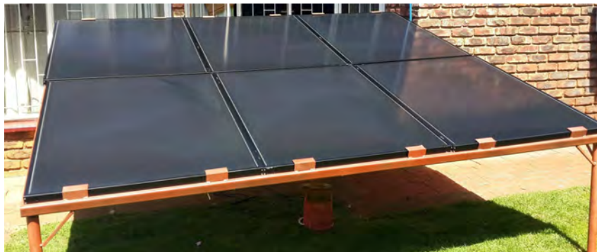
Figure 5-8: Installed array of solar PV panels
