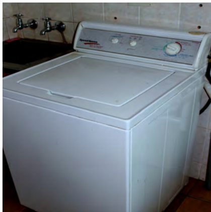
(a) Installed washing machine
