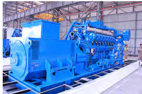
(b) HFO genset
