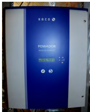
(a) Installed Powador 2002 GTI
