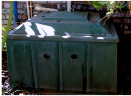
(a) Swimming pool pump enclosure
