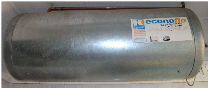
Figure 5-2: 150 litre, 3 kW installed geysers
