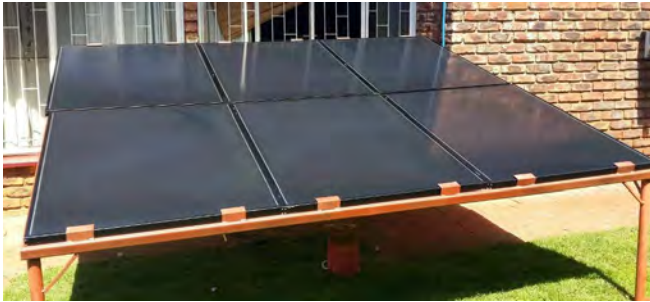
Figure 6. Installed PV modules
