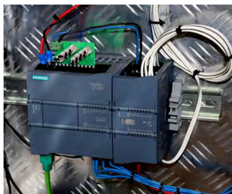
(a) Installed Siemens S7-1200 PLC
