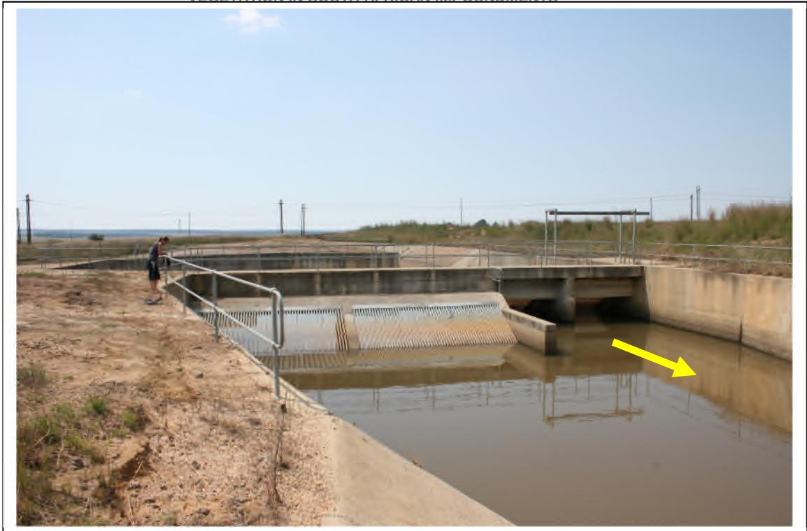
PLATE 5.24 Stainless steel grids on the inflow structure Geelhoutboom balancing dam preventing grass carp from escaping from the Geelhoutboom Dam upstream into the Geelhoutboom Canal. Direction of flow is indicated by the yellow arrow.
