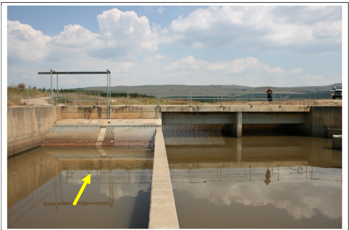
PLATE 5.25 Stainless steel grids on the tail end structure of Geelhoutboom Canal preventing debris from entering Geelhoutboom Dam (flow direction towards the grids on the left). Direction of flow is indicated by the yellow arrow.
