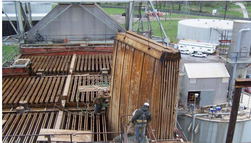
Figure 3. 1: Replacement of discharge and collecting electrodes
