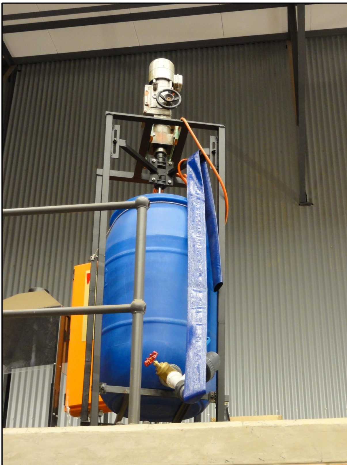
Figure C-10: Photo – Coal slurry tank with agitator motor and shaft
