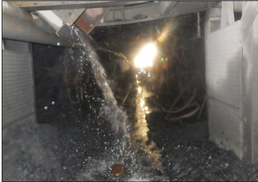
Figure 3-11: Water flowing out of box fronts and XC conditions
