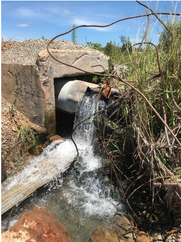
Figure 4. 6: Groundwater sample: Ruptured extraction pipeline from a shaft (Researchers personal library).
