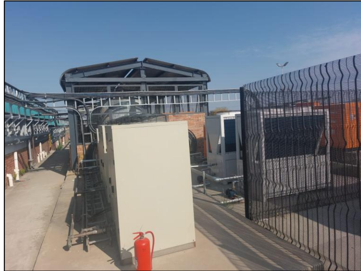
Figure 11: Change house heat-pump installation for case study EEP A
