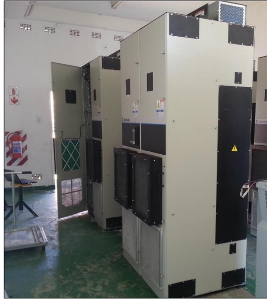
Figure 71: 400kW VSDs installed on the condenser and evaporator water pumps of Mine A.
