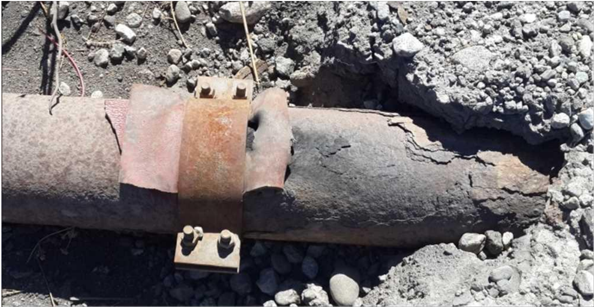
Figure 9: Poorly repaired air leak at platinum Mine A.
