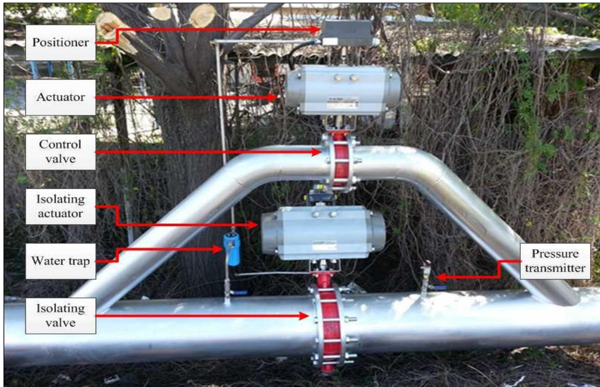
Figure 11: Surface control valve utilised on Mine A.
