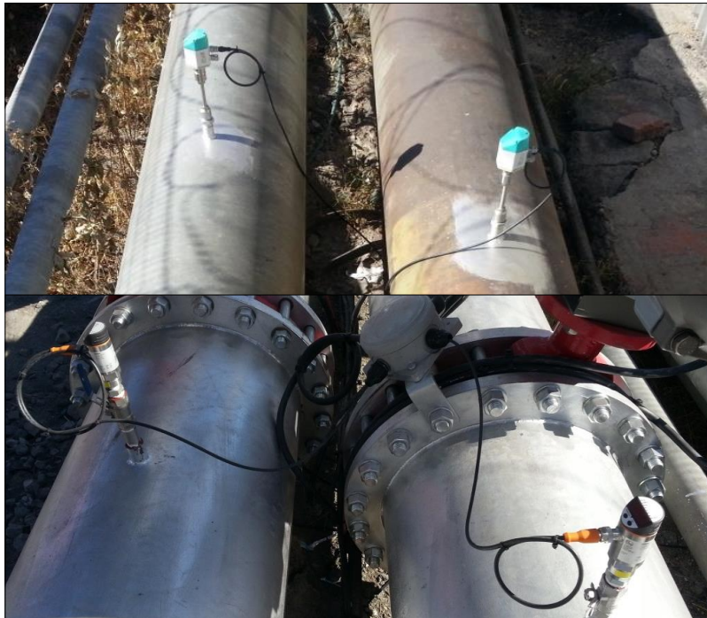
Figure 61: Air mass flow meters and pressure transmitters installed on Mine A compressed air system.
