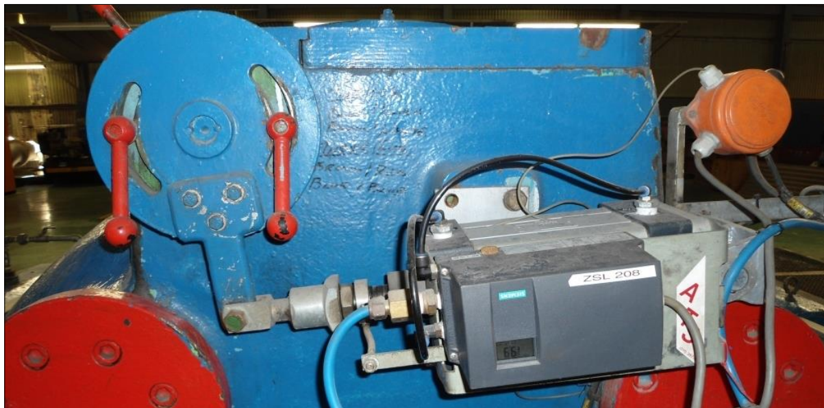
Figure 63: Pneumatic actuated inlet guide vane controller of Compressor 1 at Mine A.
