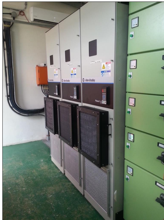
Figure 70: 200 kW and 250 kW VSDs installed on the condenser and evaporator water pumps of Mine A.
