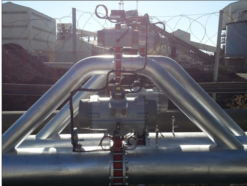
Figure 60: Downstream control valves installed on Mine A compressed air system.
