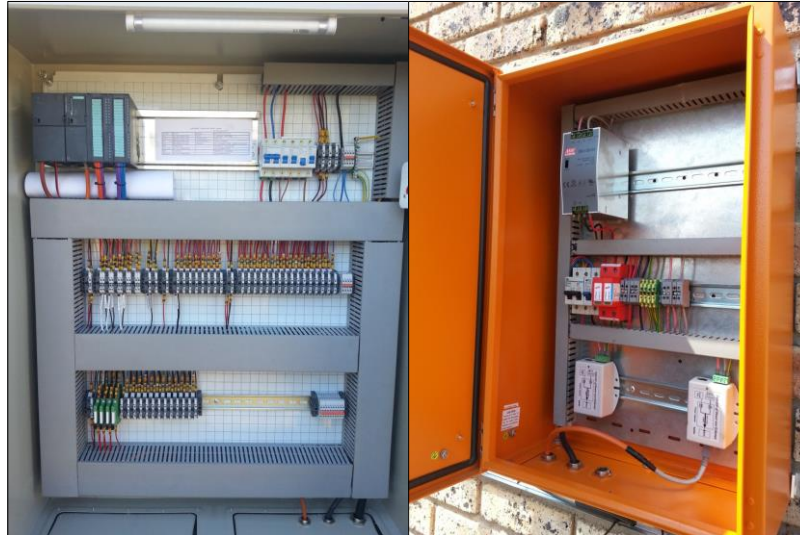
Figure 62: PLC unit installed on Mine A compressed air system.
