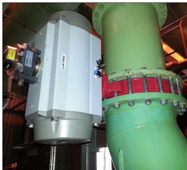
Figure 69: Pneumatic actuating control valve installed on the condenser water cycle of Mine A.
