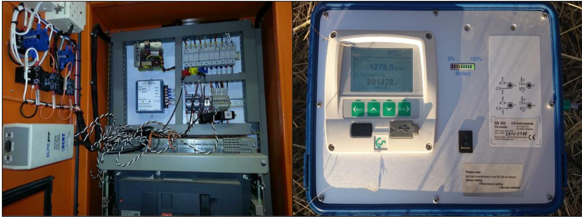
Figure 28: Temporary power and air flow loggers.
