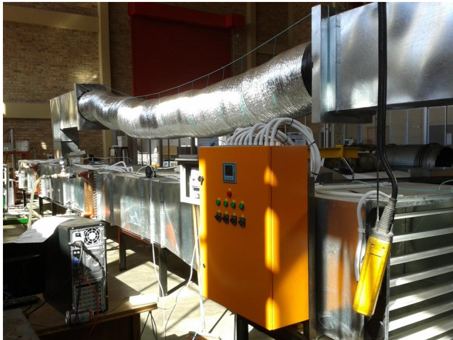
Figure 18: Photos of the coil-testing tunnel at the NWU.
