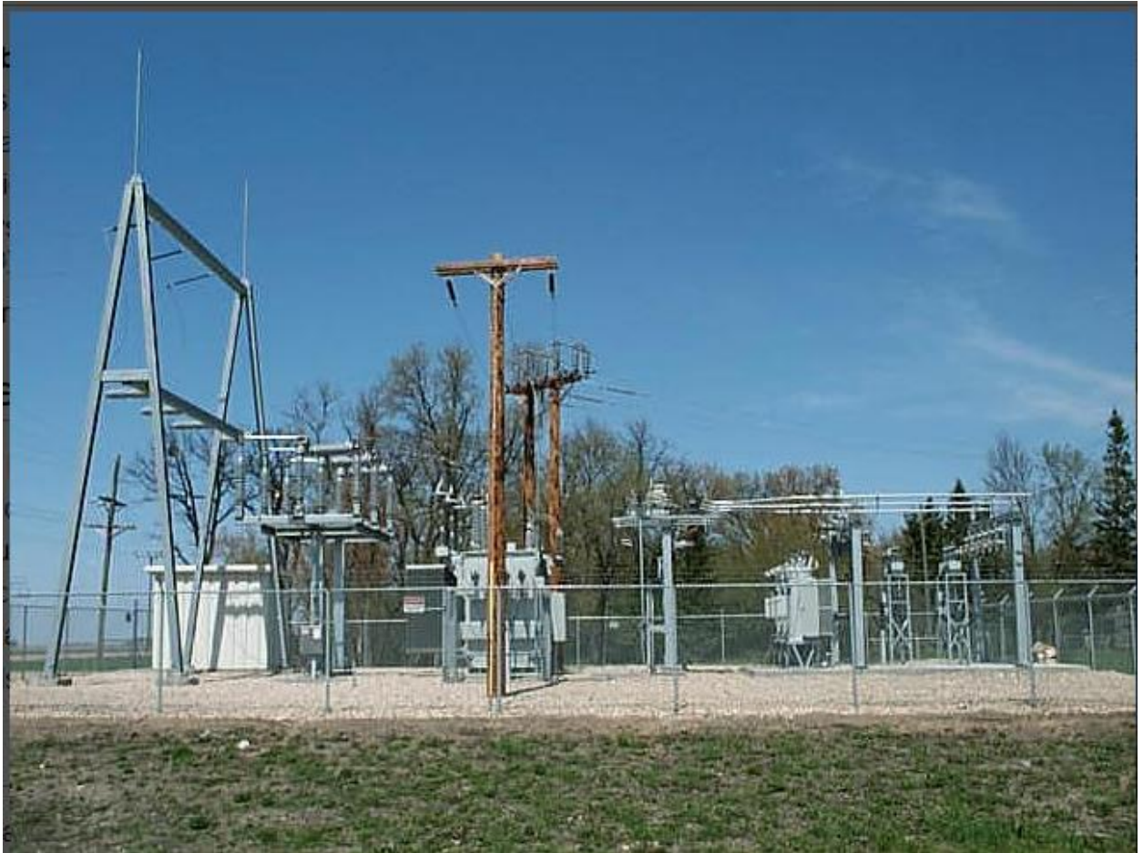
Figure 4: Example of smaller substation (Energy Education, 2022)
