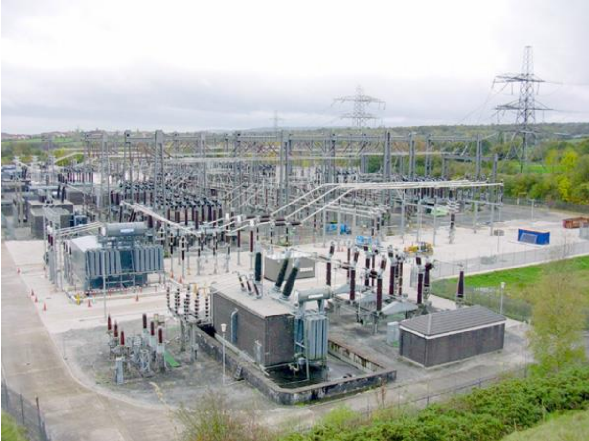
Figure 3: Example of bigger substation (Energy education, 2022)
