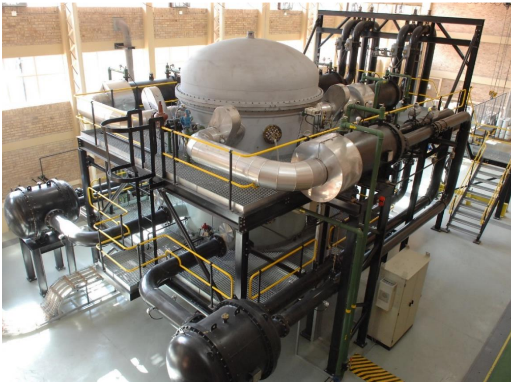
Figure 2.5: A photograph of the HTTU facility at the Potchefstroom Campus of the North-West University.
