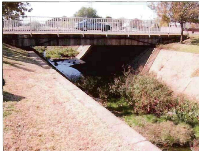
Figure 2.5 Wasgoedspruit upstream of the Van Riebeeck Street bridge in the Central Area in Potchefstroom.
