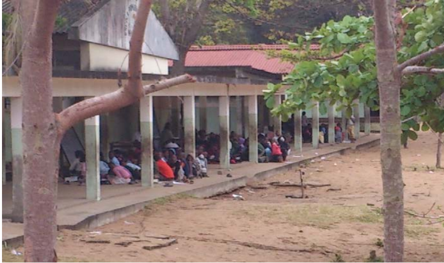
Photo 1: Local school in Bilene – dilapidated infrastructure
