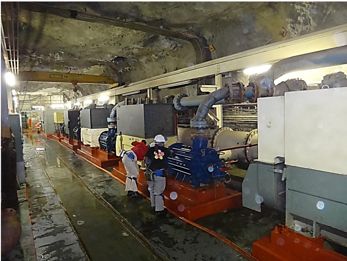
Underground pumping station 4
