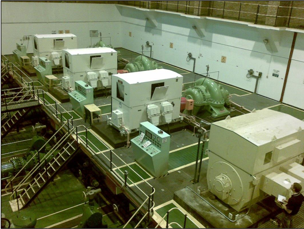
Rietfontein pump station near Kriel
