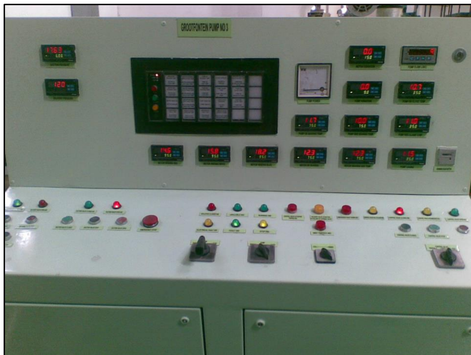
Figure 28: Grootfontein relay logic panel
