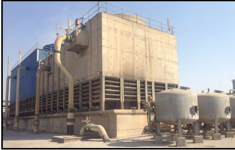
Figure 4.12: HDPE/Granulation plant cooling tower with sand filter system
