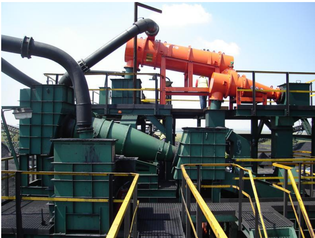
Figure 4.22: Pump fed 3 product cyclone installed at Umlalazi Colliery (De Korte, 2012)
