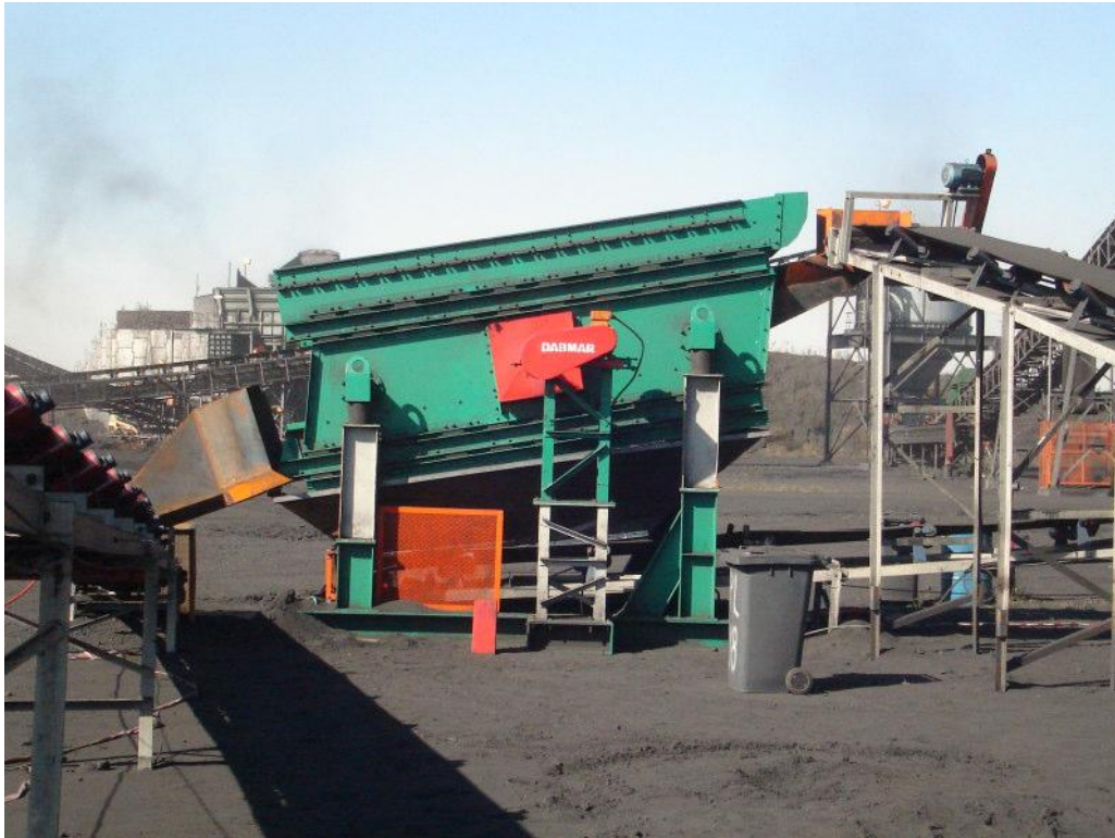
Figure 4.17: Bivi-TEC screen installation at Leeuwpan (Lundt et al, 2007)
