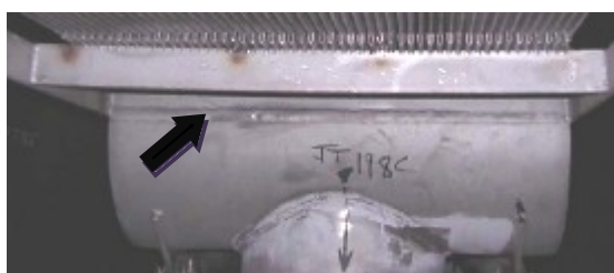
Figure 6: A photograph of the bottom header showing the weld line where the two halves of the header were welded together. The bottom guide frame and u-shaped guides are also visible
