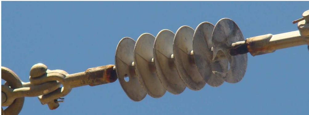
Figure 2-6 Insulator failure on the FJM 22 kV line due to sustained fault across insulator sheds
