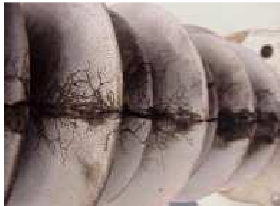
Figure 2-7 Tracking across sheds of insulator [2]
