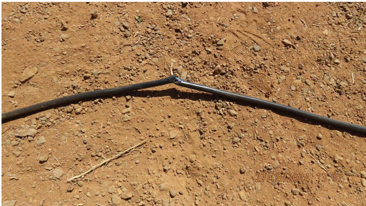
Figure 51: Damaged power cable
