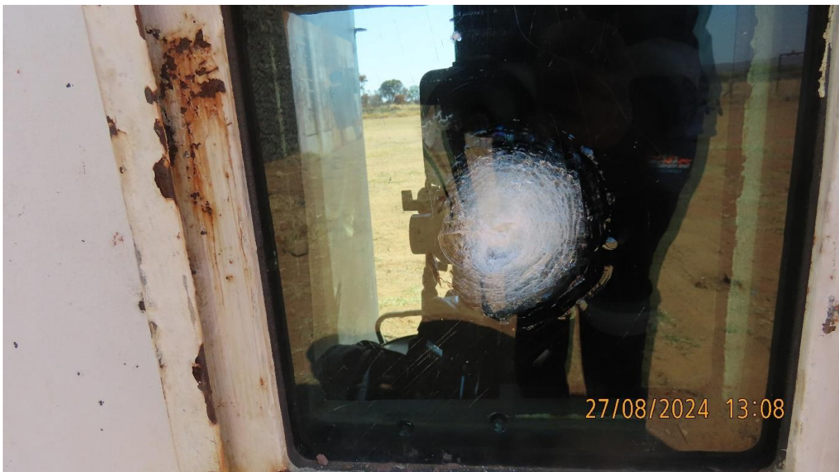
Figure 53: Damaged protective glass
